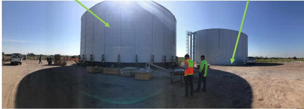
Raw water tank
